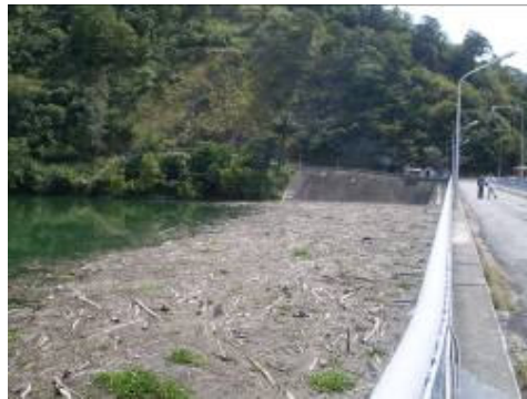
Build up of debris and mud and silt leading to the actual spillway of the dam, Luzon, Philippines.
